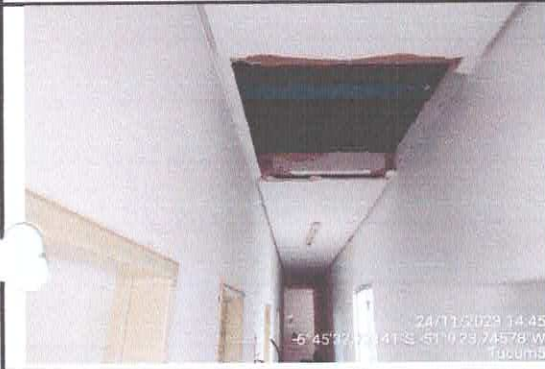
FORRO A RESTAURAR
